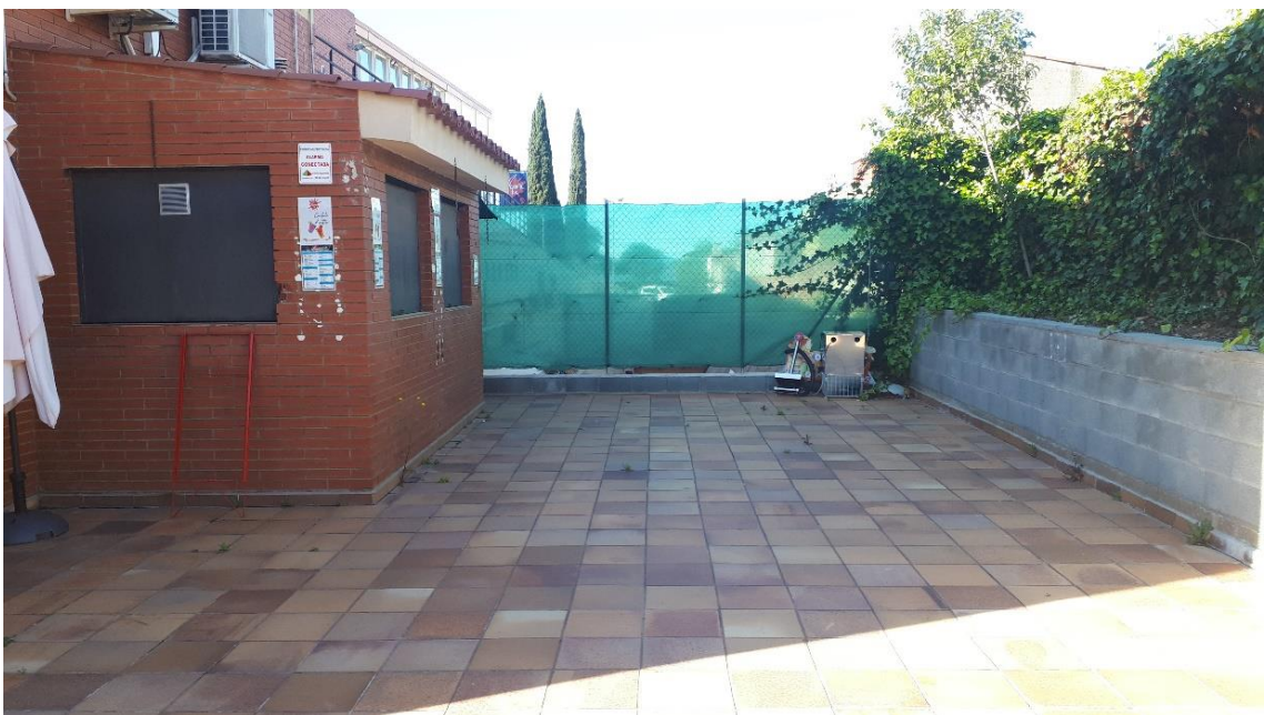
Coberta sala instal.lacions P2
